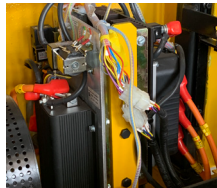
Rear mounted controller for easy maintenance
